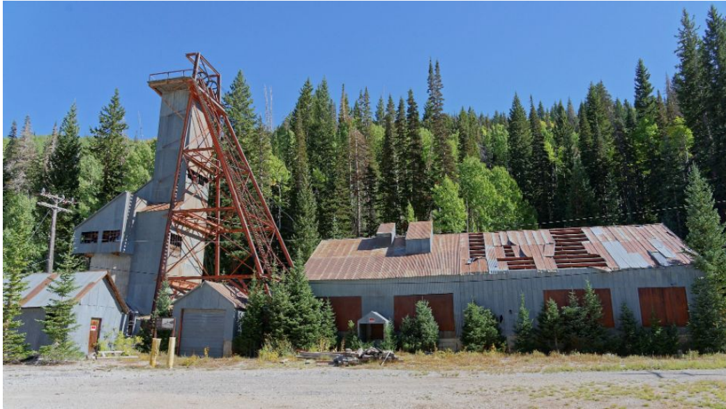
Thaynes Headframe & Hoist House in October 2022. The roof on the building right of the headframe legs has been damaged.
