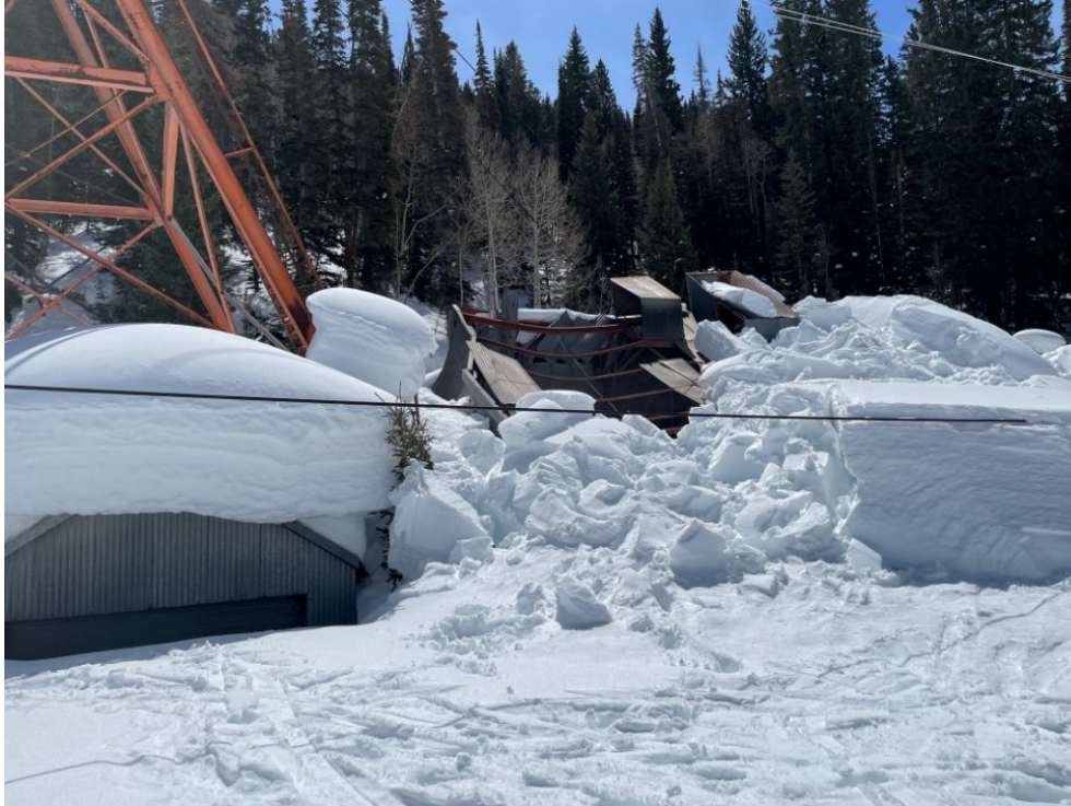
South Side (front). The entire roof of the hoist house (right of the orange headframe) has collapsed due to snow load.
