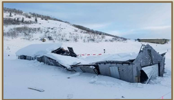
Silver King Warehouse - Collapsed in 2019
