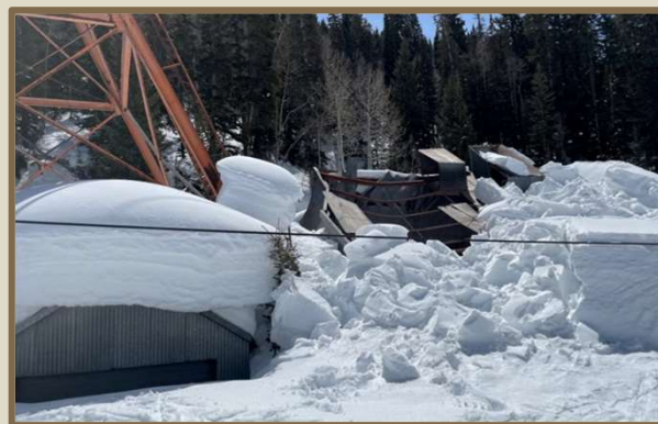
Thaynes Hoist House - Collapsed in 2023
